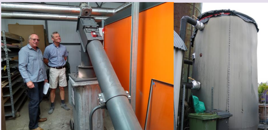
Case Study 1 – Large Greenhouse-Retail Space
